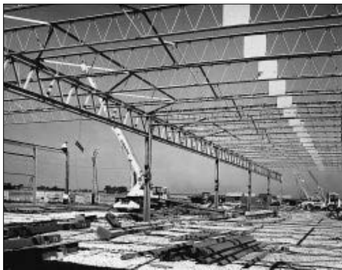
Fig. 5.16 Single-storey steel framework. Although some of the structural connections here are rigid, the majority of the horizontal elements have hinge joints. The regularity of the arrangement and the presence of a triangulated bracing girder in the horizontal plane (top left) are typical of a discontinuous framework. (Photo: Photo-Mayo Ltd)
