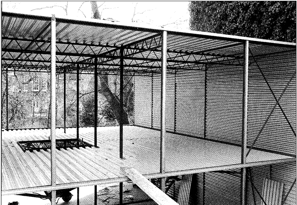
Fig. 3.13 Hopkins House, London, UK; Michael Hopkins, architect; Anthony Hunt Associates, structural engineers. The floor structure here consists of profiled steel sheeting which will support a timber deck. A more common configuration is for the profiled steel deck to act compositely with an in situ concrete slab for which it serves as permanent formwork. (Photo: Pat Hunt)
